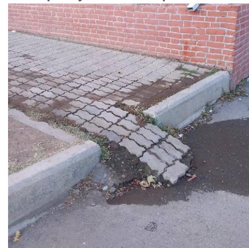
Poor quality access ramps.
