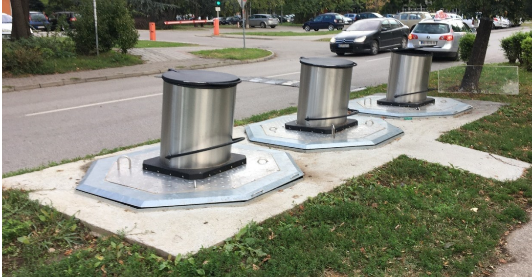
Figure 26 Underground waste collection points
